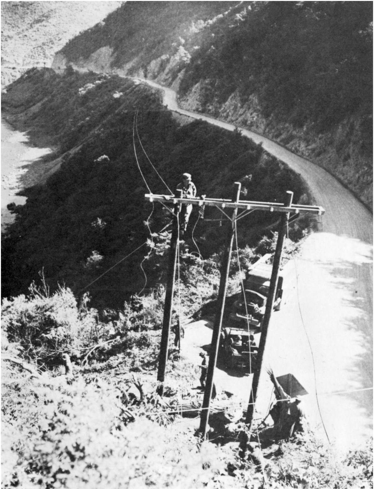
SIGNAL CORPS MEN REPAIRING COMMUNICATIONS LINES in a mountain pass south of Hwach'on.
